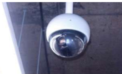
(3) CCTV in a storage space
